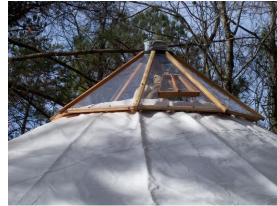
A sky-light sets on the very top. A chimney pipe will go through it.
